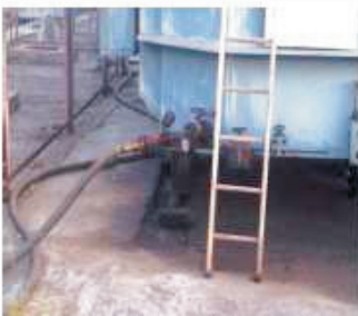
Inlet to Plant View at Transformer Bottom Valve
