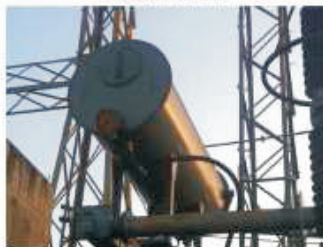
Outlet from Plant View at Conservator Bottom Valve
